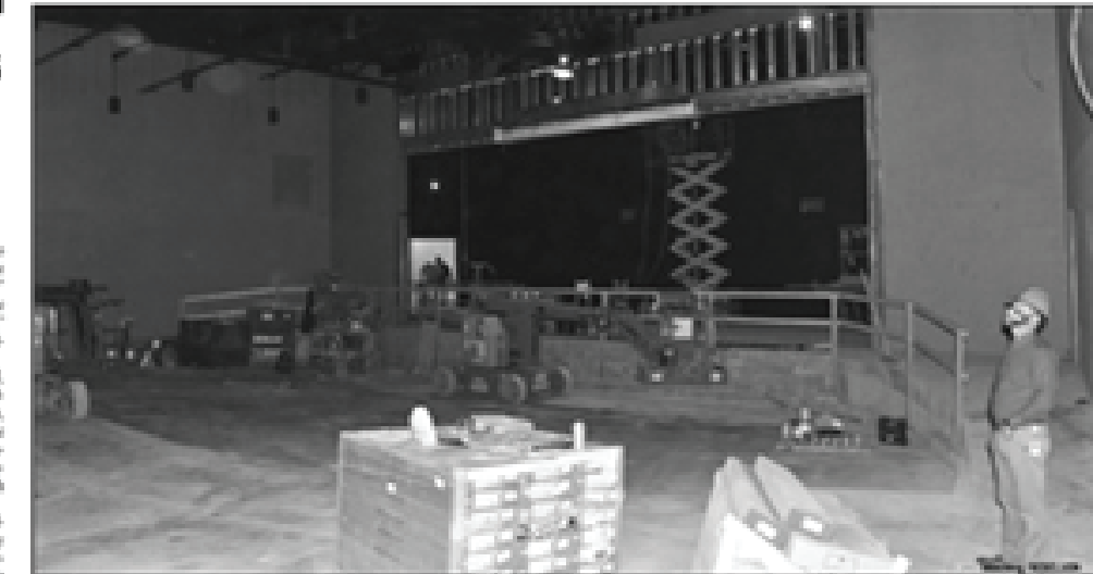
Principal Timothy Schlotman observes the progress on the performing arts center construction on Nov. 21. The 400-seat space is expected to be completed in February and should host its first events in the spring.
